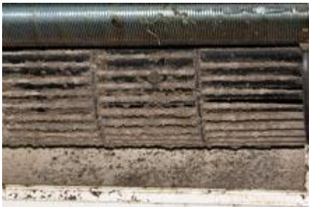
Mold Growth on Blower Wheel
