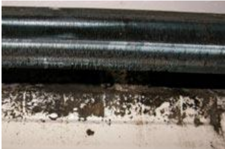
Mold Growth Before UV Installation
